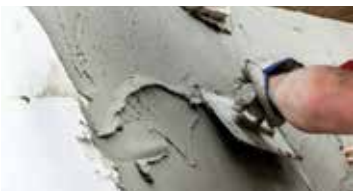
DryMix Building Materials Processing
